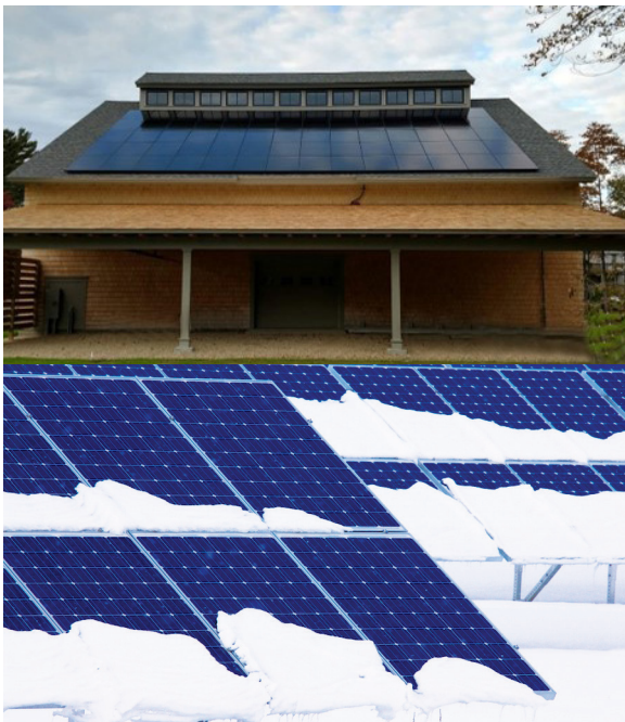
Figure 1: Dormer shading, photo courtesy of Mass Renewables (top); shading from partial snow coverage (bottom).
